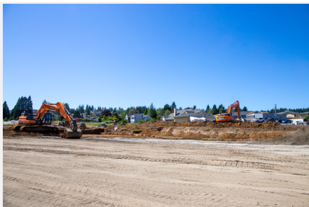
MAIN PIC: Crews continue their work on Good Shepard Village in Happy Valley on June 23. (Staff photo by Alex Jensen)
