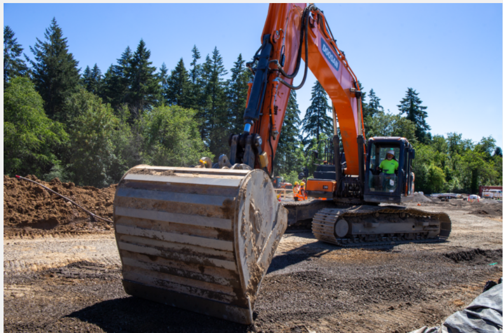
A crew member with Lauzon Contracting backfills a newly placed storm water line for the Southeast Skyshow Place extension at Good Shepard Village in Happy Valley on June 23. The $60 million development will have 143 affordable apartments when complete in late 2023. (Staff photos by Alex Jensen)
